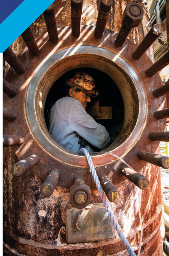
Tower Technician Pedro Chavez bolts a tray inside a hydrolyzer tower before final closure at the BASF plant in Beaumont, Texas. Photos/Nick Grancharoff
