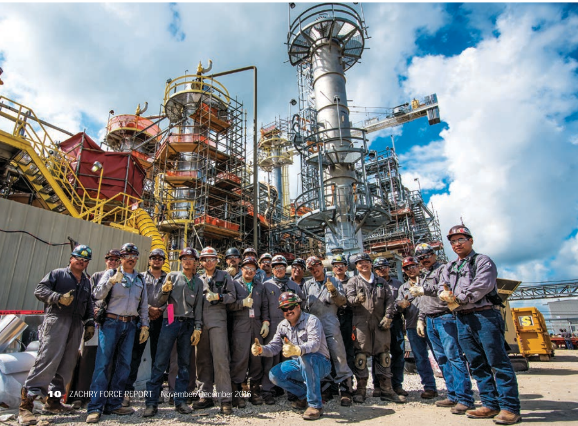
Tower Services Superintendent Rick Cervantes and his crew of 21 technicians worked on numerous vessels this year—blinding them for entry, opening, cleaning, inspecting and installing equipment—at the BASF plant’s Dicambria Unit in Beaumont, Texas. The tower work was part of a large turnaround that included JVIC pipefitters and Zachry scaffolding crews.
